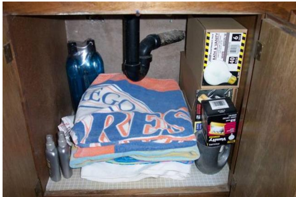
Figure 2. Good storage of dry materials in sink cabinets.
