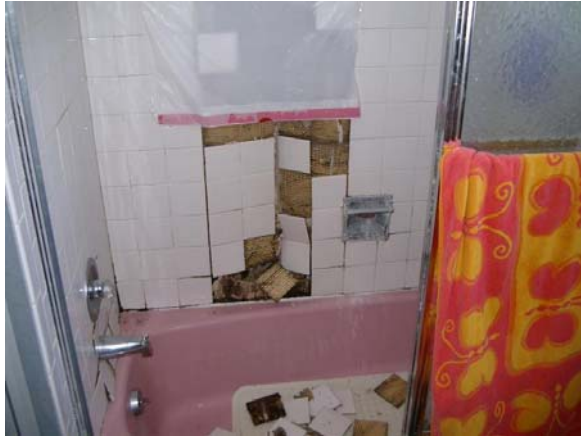
Figure 3. The result of deteriorated grouting and caulking.
