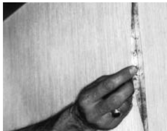
Mold and mildew aren't always obvious. This extensive mold growth is only apparent when the vinyl wall covering is peeled back. Impermeable wall coverings such as this can often worsen a mold problem by trapping moisture between the interior finish and the gypsum board.
