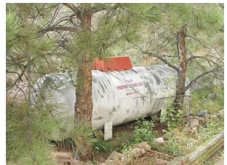
Example of a poorly maintained propane tank pad area.
