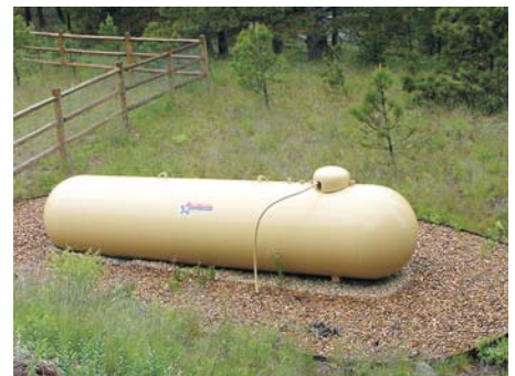
Example of a proper propane tank installation.
