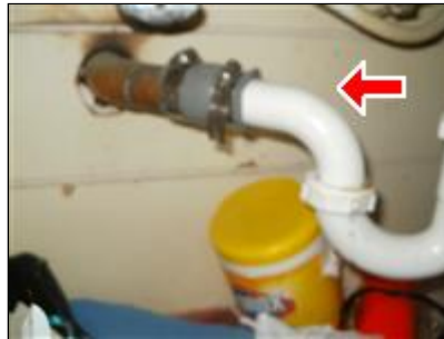
8.0 Picture 1 prior repair
