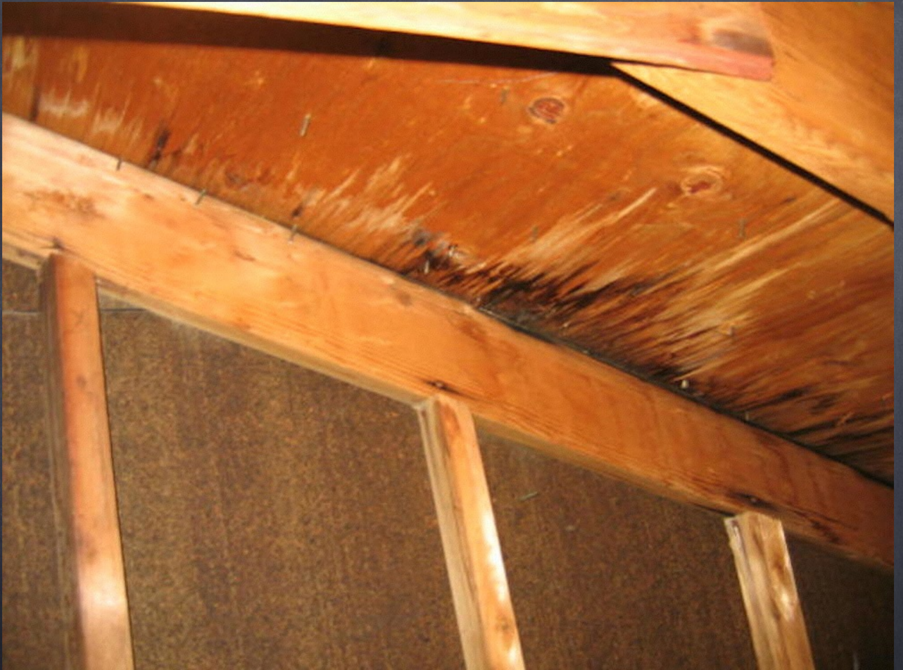
Roof leak at chimney flashing
