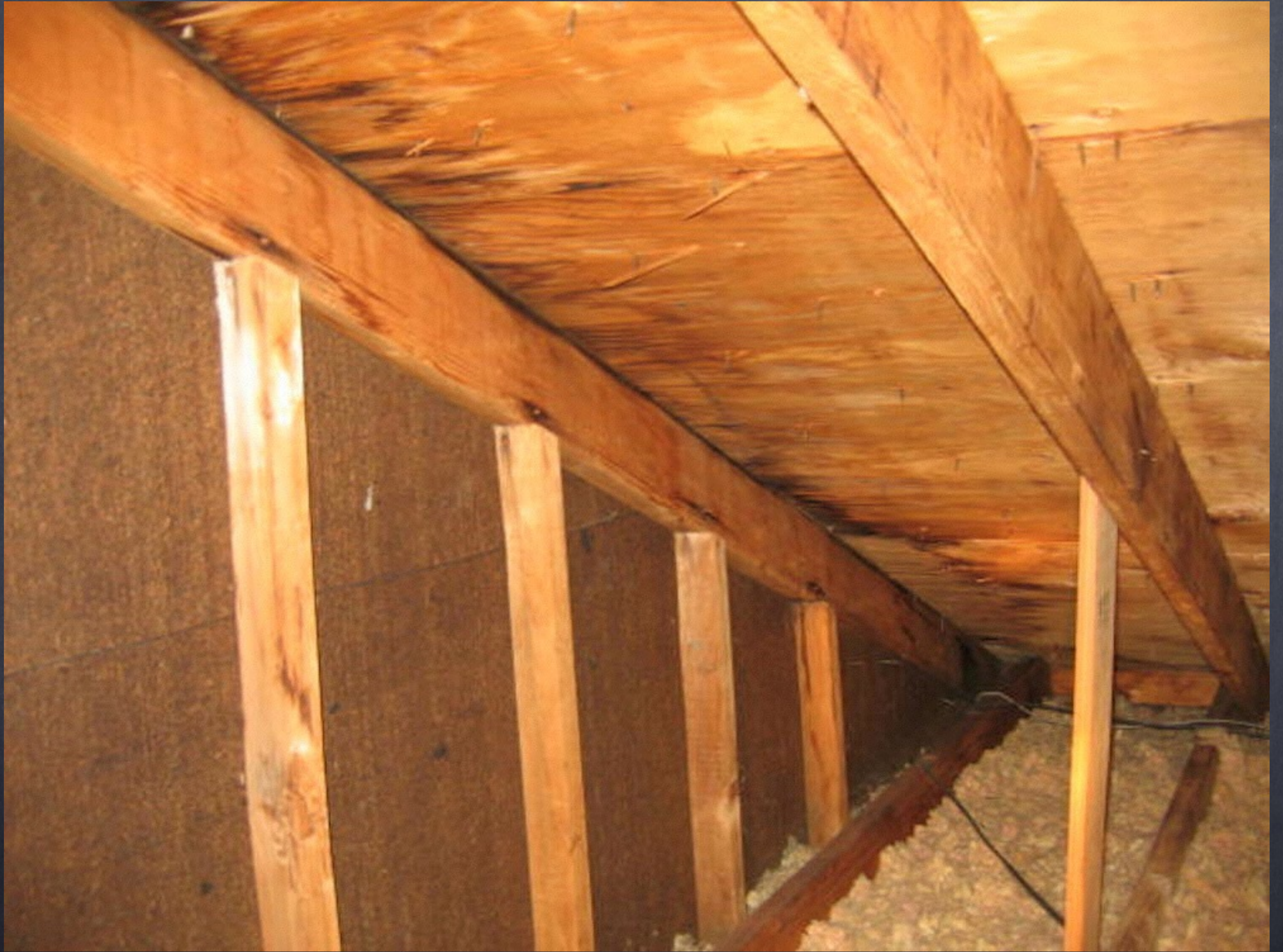
Roof leak at chimney flashing
