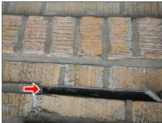
2.0 Picture 2 Front Parapet Wall mortar joints loose and falling out
