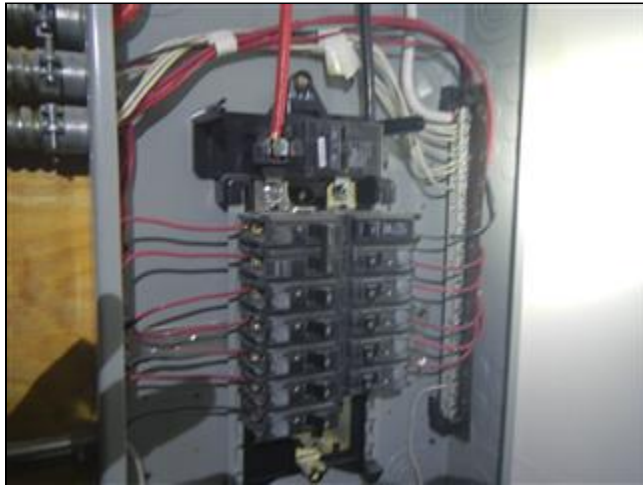
8.6 Picture 1 First Floor Sub Panel
