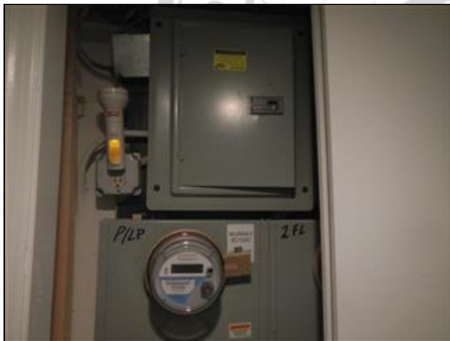
8.6 Picture 2 Common area Panel
