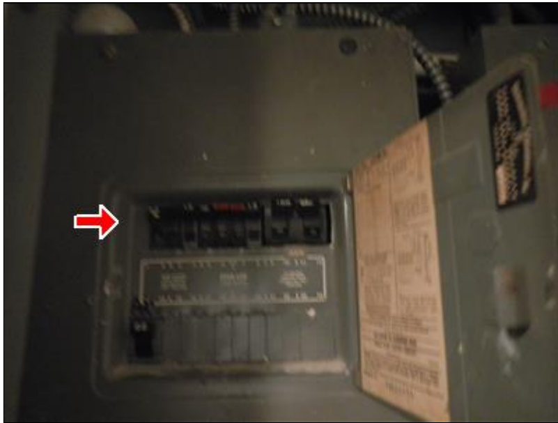
8.1 Picture 1 Federal Pacific Sub Panel
