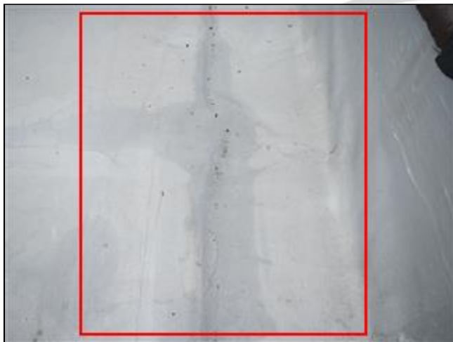
1.0 Picture 2 Water bubble under roof covering at left rear corner of roof
