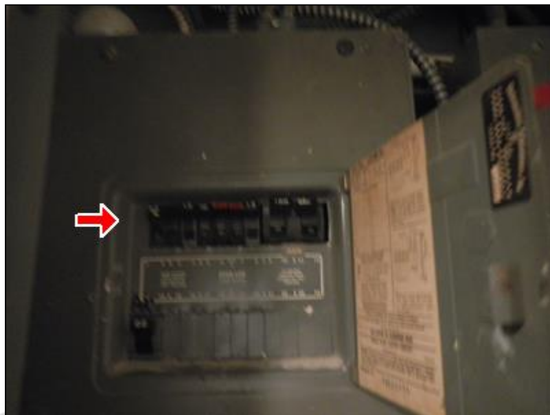
8.1 Picture 1 Federal Pacific Sub Panel
