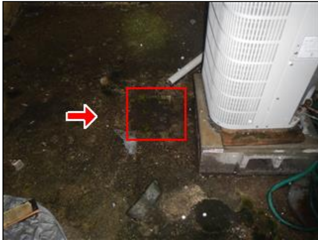
2.3 Picture 1 Drain clogged in mini court yard
