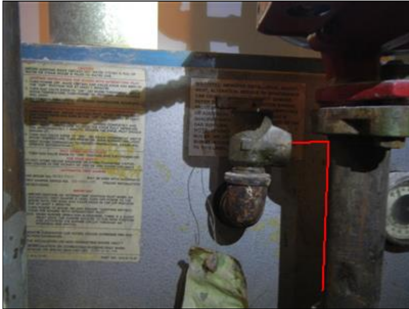
9.2 Picture 1 TPR pipe extension and elbow not installed
