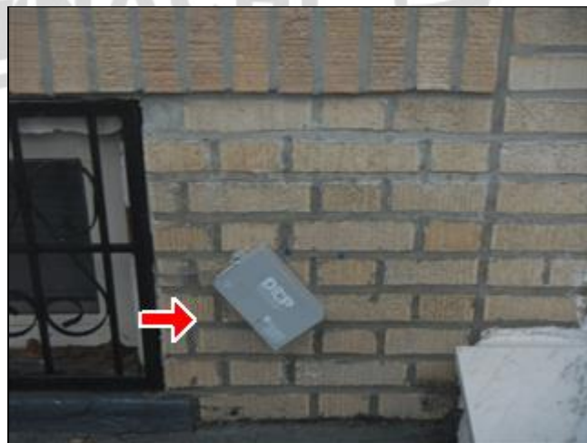
7.1 Picture 1 Remote water meter hanging off front wall
