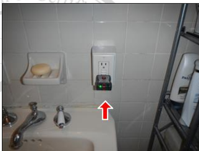
5.5.C Picture 1 GFCI outlet inoperable, open ground
