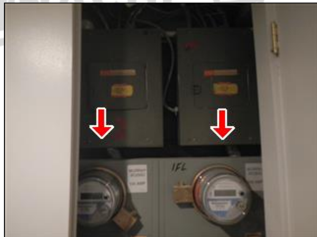
8.7 Picture 1 Electric meters
