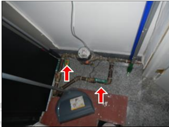
7.3 Picture 1 Main water shut off valve
