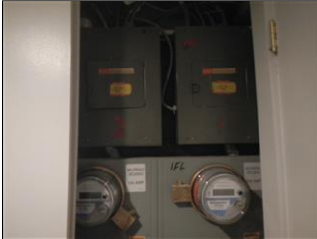
8.6 Picture 3 First and second floor Main Panels
