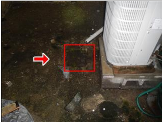
2.3 Picture 1 Drain clogged in mini court yard
