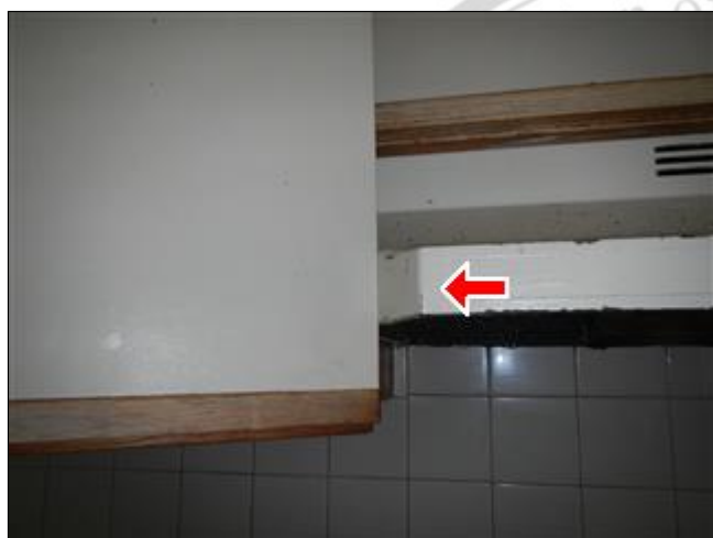
3.4.B Picture 3 Wall corner cabinet door hits range hood.
