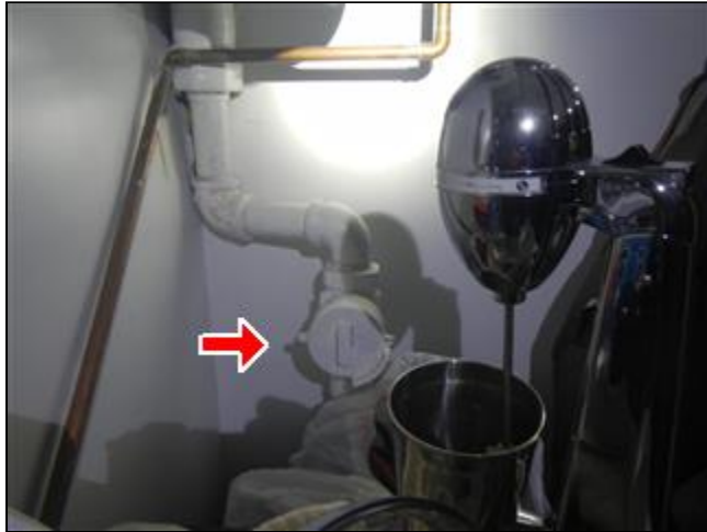
7.5 Picture 1 Main Gas Shut Off Valve
