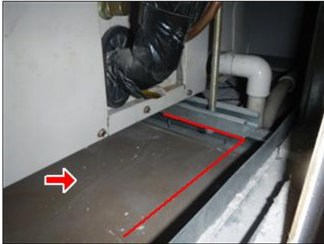
9.8 Picture 1 No condensate drip pan present under air handler
