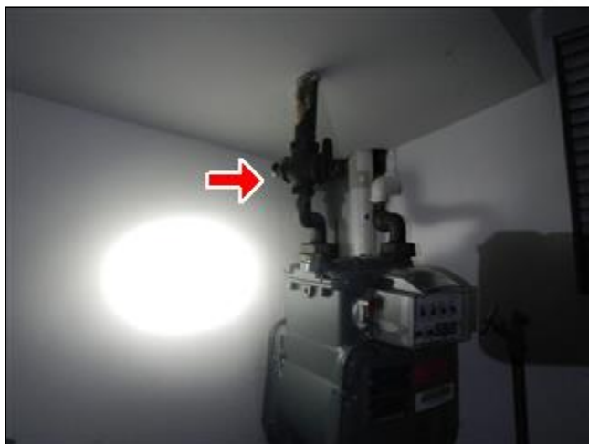
7.5 Picture 2 Gas valves at meters for each apartment
