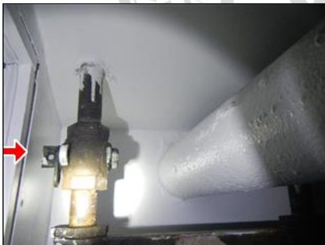
7.5 Picture 3 Gas valves at meters for each apartment
