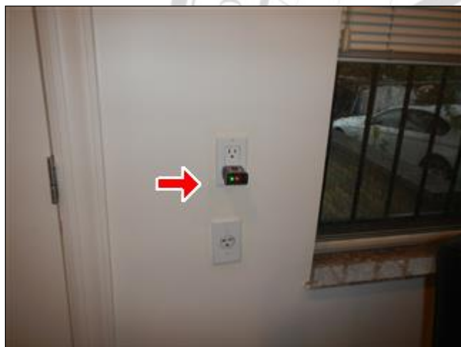
4.6.C Picture 1 Outlet on rear wall first floor dining room has open ground
