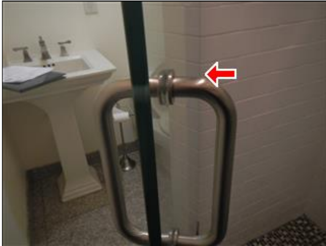
5.4.B Picture 1 Door handle loose to glass shower door
