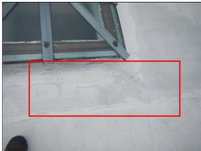
1.0 Picture 1 Water bubble under roof covering at rear corner of sky light
