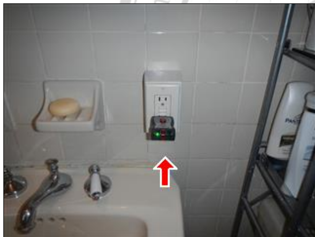
5.5.C Picture 1 GFCI outlet inoperable, open ground
