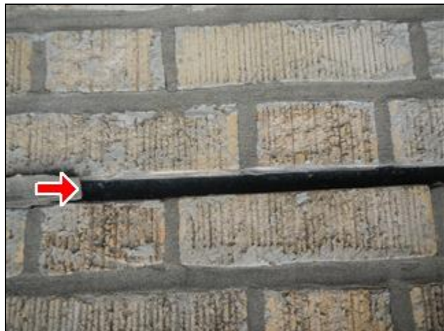
2.0 Picture 1 Front Parapet Wall mortar joints loose and falling out
