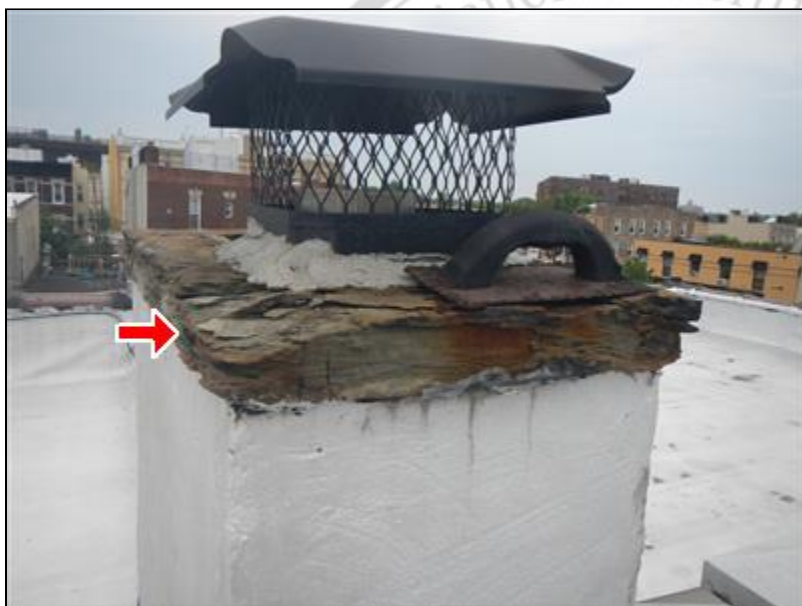
1.2 Picture 2 Chimney blue stone cap is badly deteriorated
