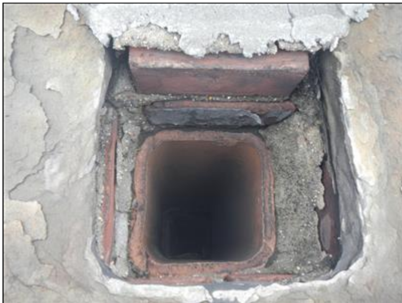
1.2 Picture 1 Ceramic Flue pipe for water heater is 6" too short.
