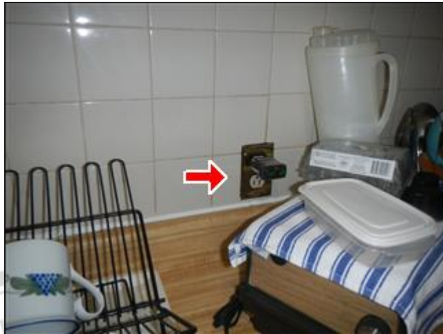
3.7.B Picture 1 Outlet to right of sink open ground and not GFCI protected
