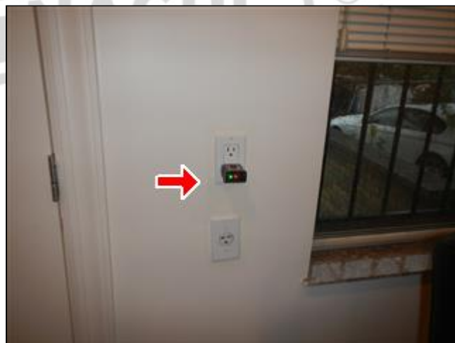
4.6.C Picture 1 Outlet on rear wall first floor dining room has open ground
