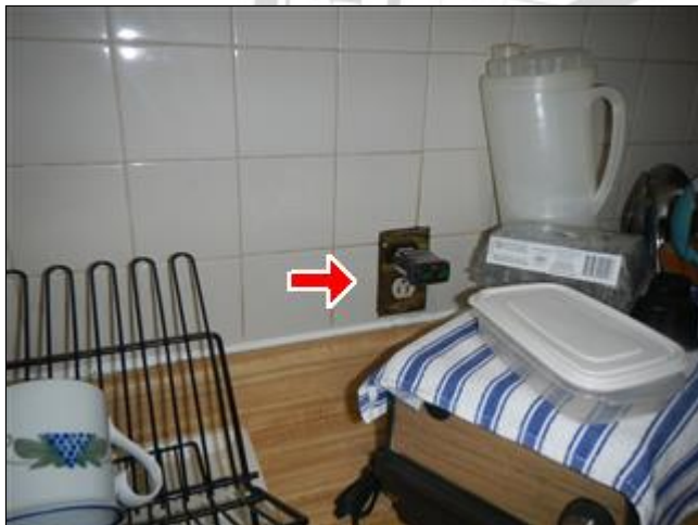
3.7.B Picture 1 Outlet to right of sink open ground and not GFCI protected
