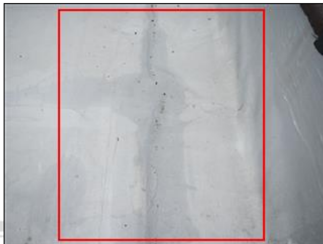
1.0 Picture 2 Water bubble under roof covering at left rear corner of roof
